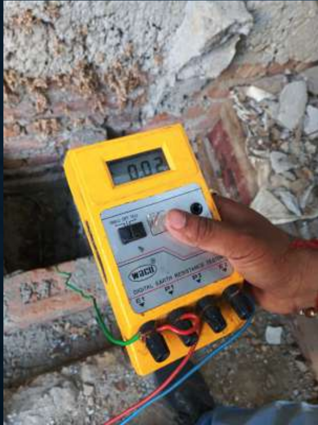
Digital Earthing Testing
